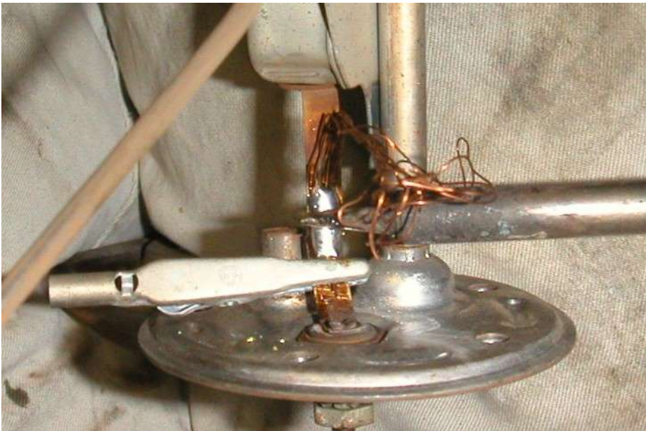
Photo 3 – Soldering a length of stranded wire in place, using an alligator clip as a clamp
